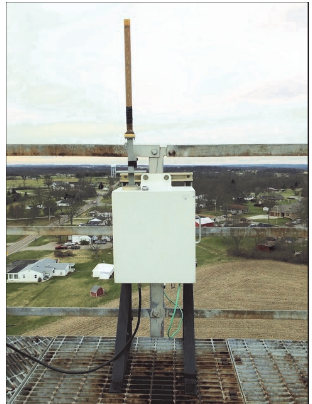
This photo shows the beacon enclosure installed on the top work platform of the tower. The enclosure mount is strapped to the railing, and the LMR400 feedline carrying the 100 MHz reference signal and DC power to the enclosure can be seen lower left. The slot antenna extends out of the top of the enclosure, clear of the railing via various fittings and adapters. Since this photo was taken, a plastic pressurization line was fitted to the AT&T waveguide adapter between the enclosure and slot array to keep moisture out of the antenna and plumbing.
